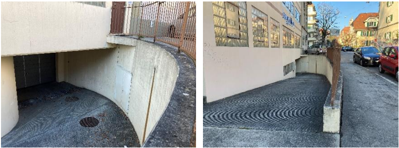
Figure 42: two pictures showing hazard area #1 (own images taken on 13.01.2022)
